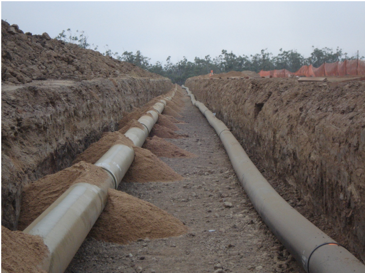
16” Ameron GRE Gas line
